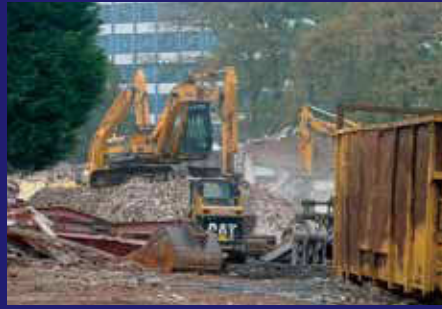
November 2008 - Looking back towards the tower block through the Somerville demolition site.
