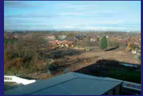
November 2008 - The site is almost clear ready for the new foundations to be laid.
